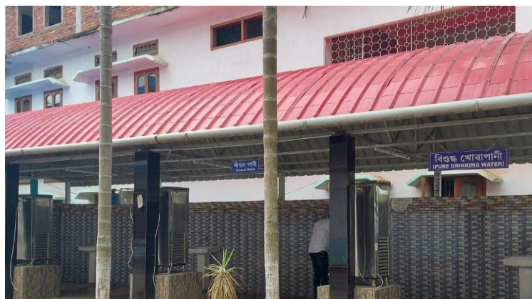
Photo 1: Water Purifiers Installed in the Campus
